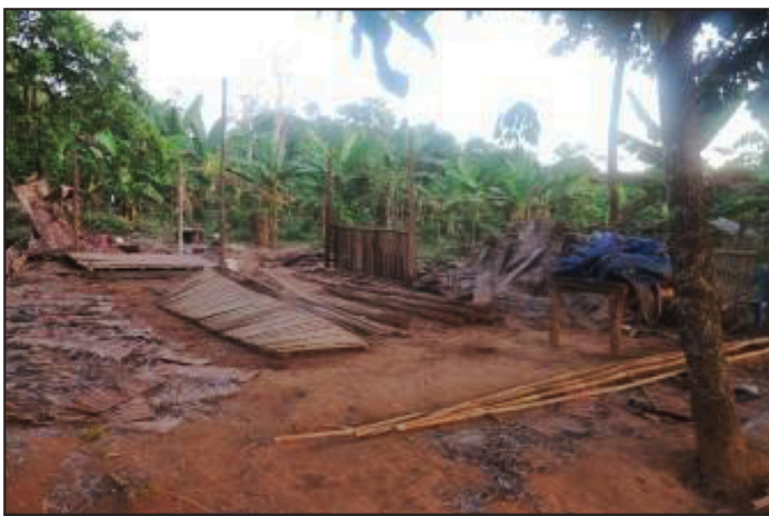
Civilian property demolished by Myawaddy Naval Base in Tenasserim Division (Case 86).
