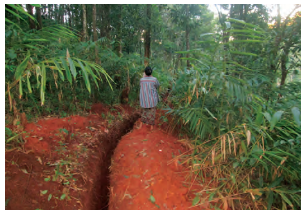
This photo was taken on November 15 th 2016 in Bl---village, Thandaunggyi Township, Toungoo District. The Myanmar Fiber Optic Communication Network Co Ltd (MFOCN) came to the area to build an underground communication cable. They did not consult the local population prior to building this cable. Because the MFOCN was granted permission by the Myanmar government, they started building the underground communication cable, digging up local land. However, some local villagers were not satisfied because their lands and plantations were destroyed due to digging. [Photo: KHRG]
