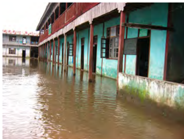
The above photo was taken on August 7 th 2012 and shows the flooding of Pa Deh Kaw High School in Nyaunglebin District. According to the community member who took the photo, flooding can be attributed to Shwegyin dam operations and resulted in the closure of the school for over one month. 171 [Photo: KHRG]
